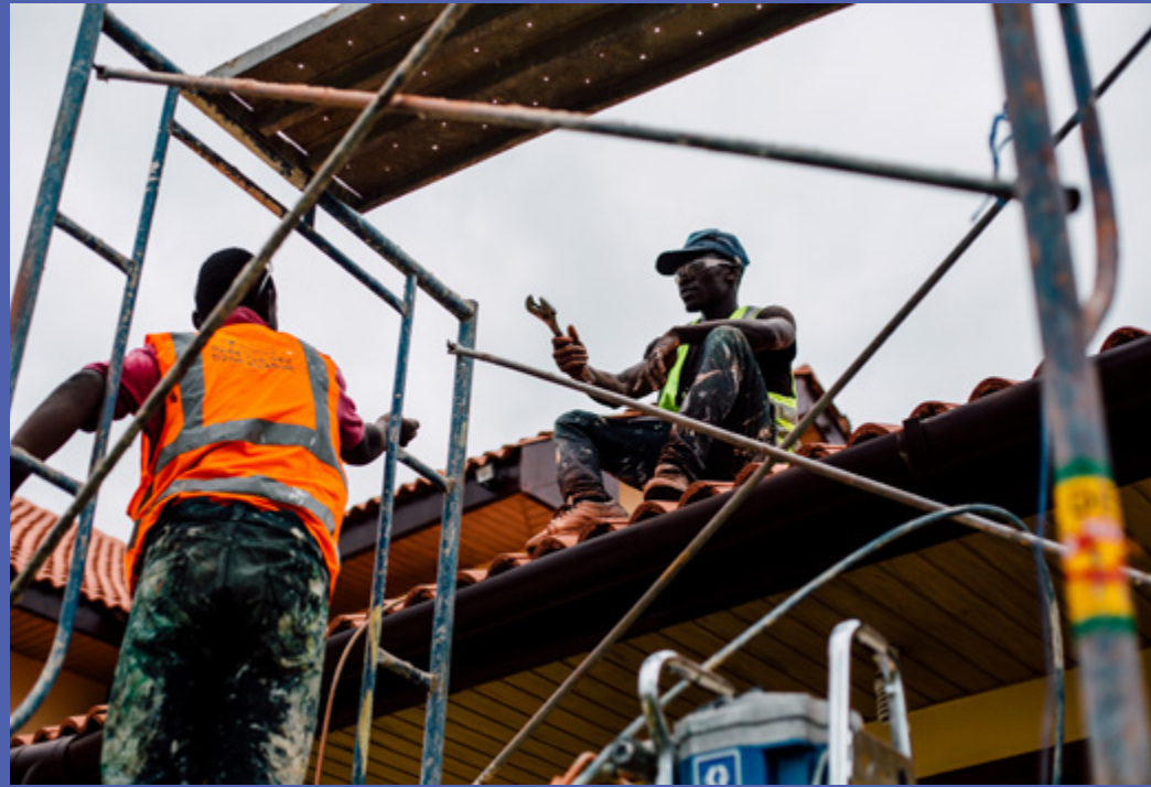
Peter Baidoo teaches one of his workers, Emmanuel Awusi, how to manage the paint-spraying machine. Emmanuel was connected with Peter through the Uniterra Program.
