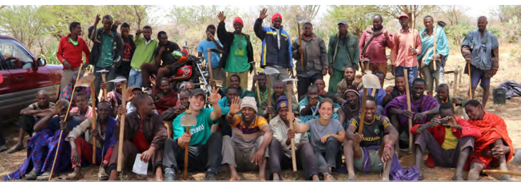
Team members Charles Bernard and Melissa Windsor with the farmers who came and dug trenches and other construction staff.
